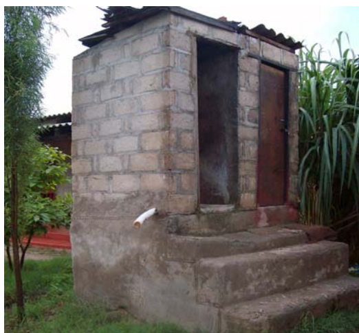
Fig.1: Overhang Pit-latrine in Madimba
